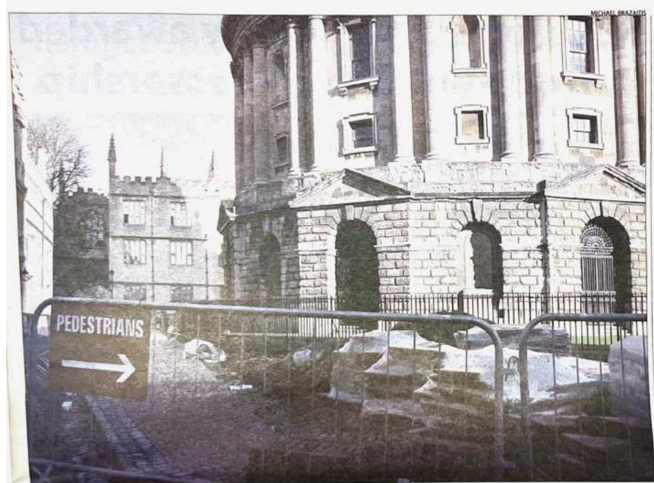
The repair of Radcliffe Square's historic cobblestones is finally underway after a year of delay, writes Sam Counsell. It will be carried out in six phases, moving round the Rad Cam in sections to reduce disruption to pedestrians. It is hoped that the project will be finished by Christmas. The cobbles and Yorkshire Paving of Radcliffe Square date back to the eighteenth century, and while patch repairs have been attempted on several occasions none have been very successful. Between 10 and 20 percent of the current stones will be reused, the rest replaced with larger river cobbles. Most of the Grade II listed Square is owned by the University, which is meeting more than half the cost of the £500,000 project. The remainder has been contributed by the City and County Councils.
